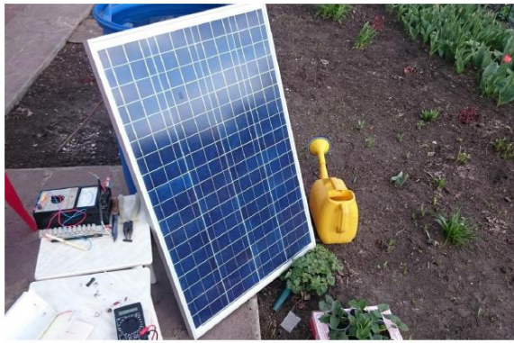
Fig.4 - Clean solar panel without film
